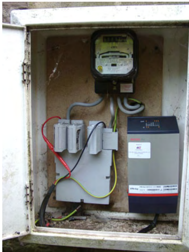
Fig. 2. The Ascom Outdoor Access Point, installed in an outdoor meter cupboard. The OAP is the unit in the lower right of the picture, and, as can be seen, was connected to the supply side of the electricity meter. (At the other Ascom-equipped premises visited there was an electrically similar arrangement, but in that case the meter and OAP were housed indoors.)
